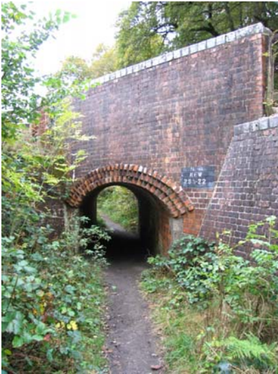
Brick Tunnel under the Par to Newquay railway line - photo Chris Tigg
